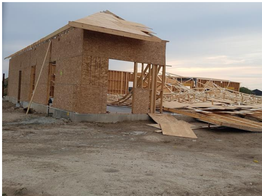
Failure of partially constructed wood-framed office in Ilderton, Ontario October 7, 2017
