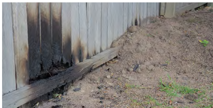
When attached to buildings, flammable fencing can cause fire spread and ignition of structures.
