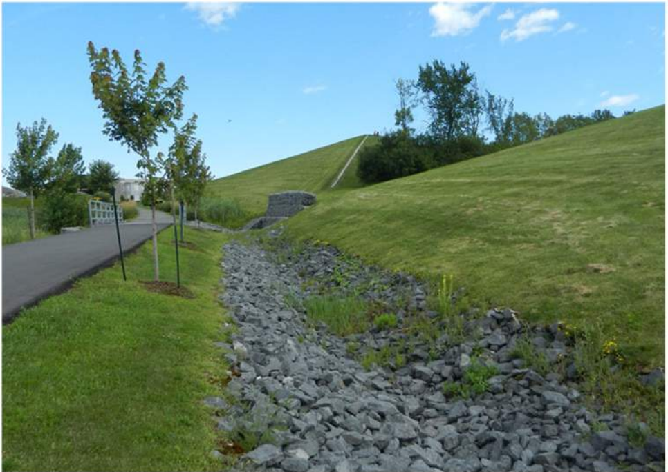
Figure 26 & 27 : Drainage pathways were created along the multifunctional corridors to connect the dry ponds to the wet ponds. (Source: ICLR)
